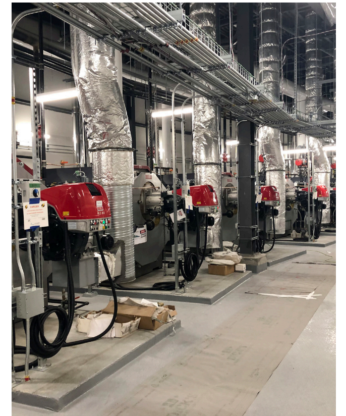
Image 16: High efficiency dual fuel condensing boilers © Ross Griffiths, Arup
